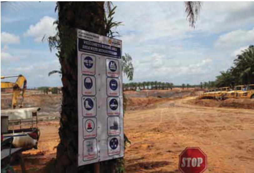
Safety signboard at site
